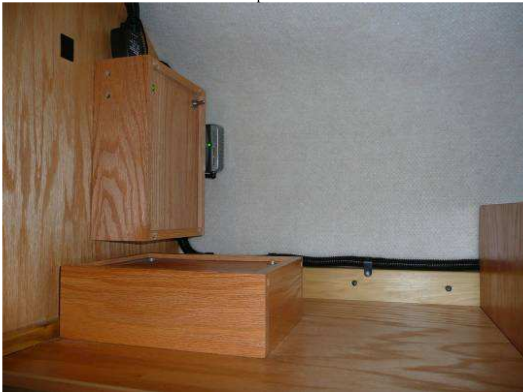
Side view as seen when cabinet door is open.
