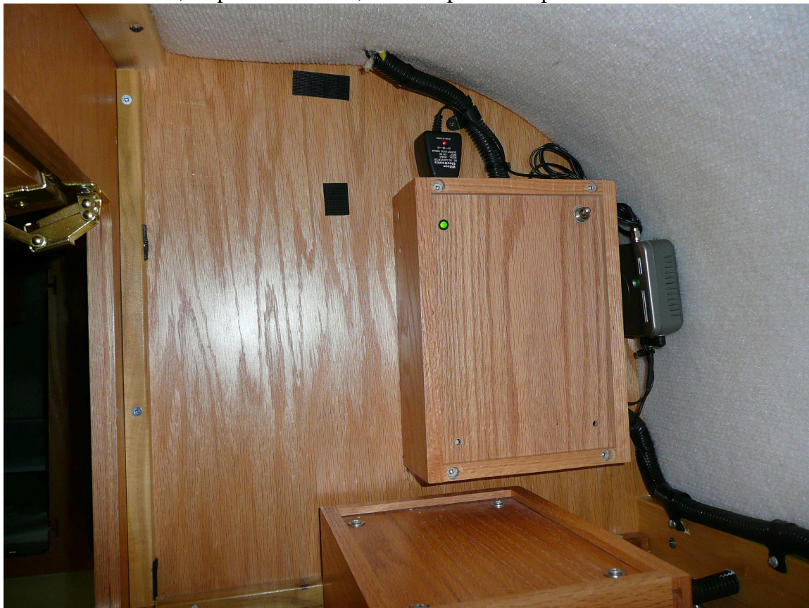
Oak cover installed, amplifier mounted, and unit powered up.
